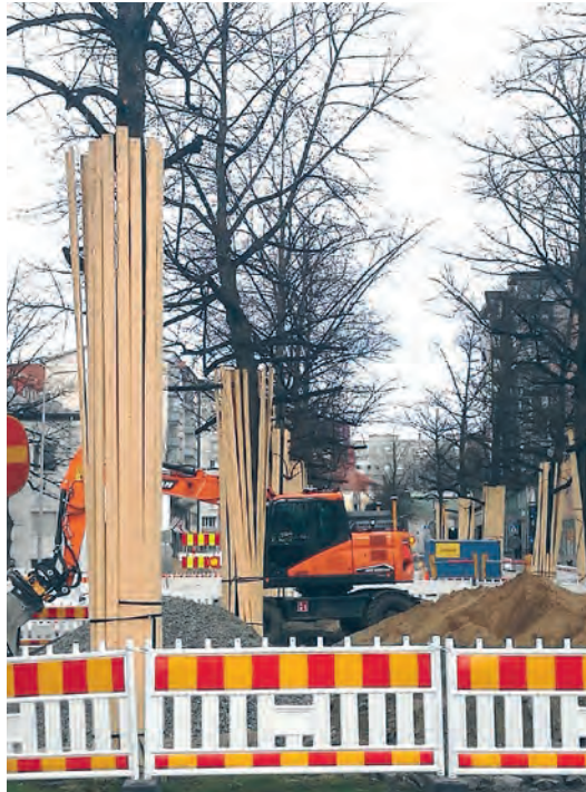
Protecting old street trees at construction sites extends their life cycle and preserves their carbon stores. (PHOTO: RANJA HAUTAMÄKI)
